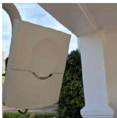
A Single Long-Range RFID Reader was Installed. PHOTO: Supplied.
